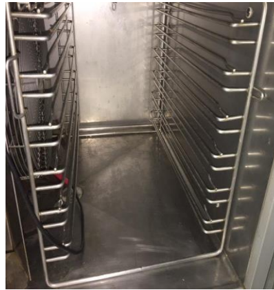
Interior of Blast Chiller
